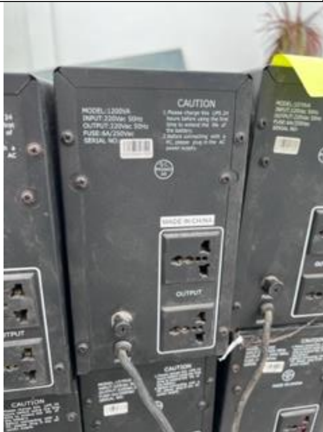
UNREADABLE UPS-BLUE GATE 1200VA
