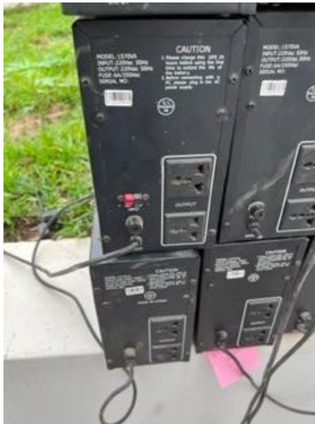
UNREADABLE UPS-BLUE GATE 1570VA
