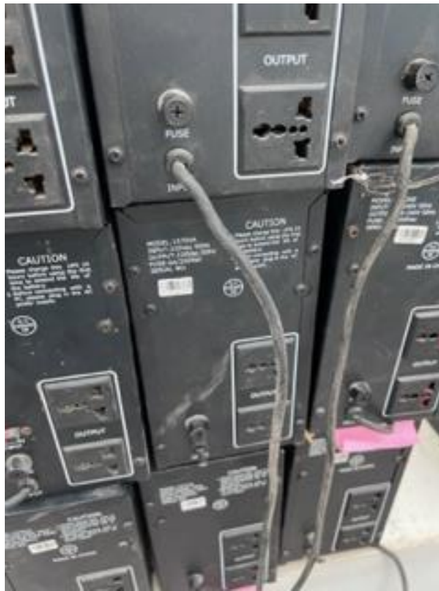
UNREADABLE UPS-BLUE GATE 1570VA
