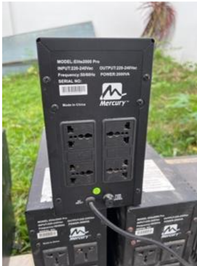
UNREADABLE UPS-BLUE GATE 1570VA
