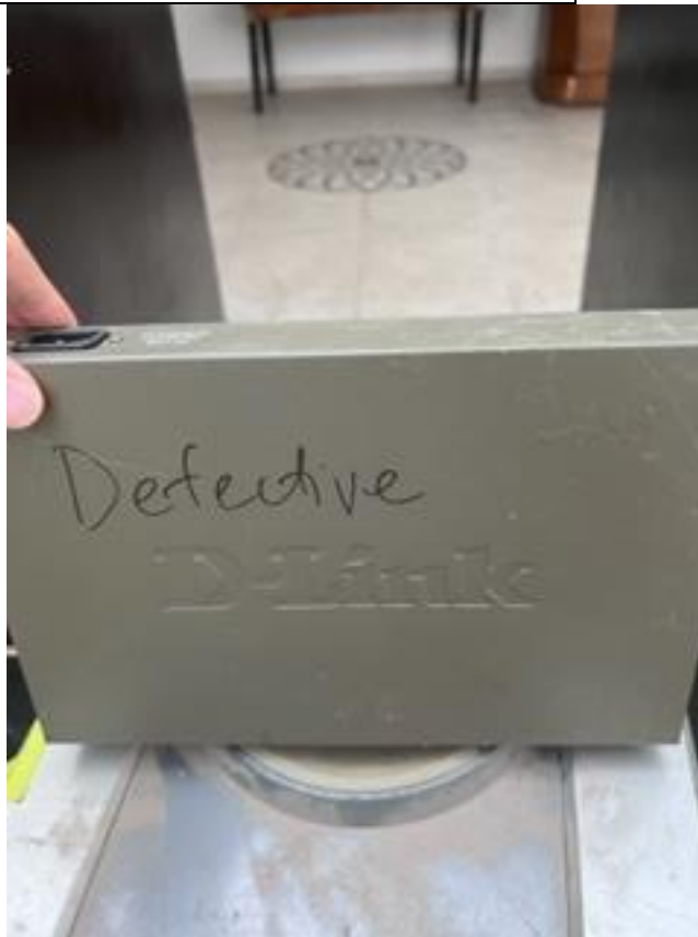
NOT FOUND ETHERNET SWITCH
