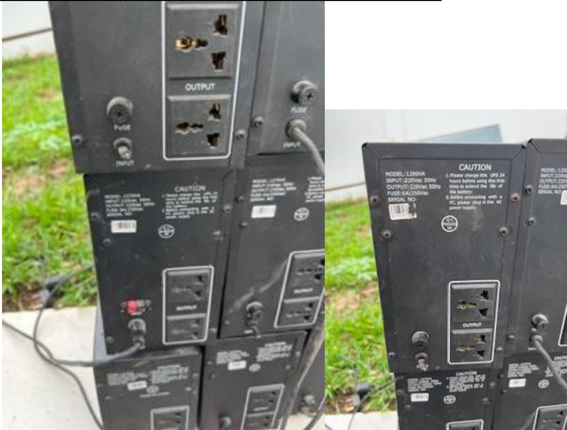
UNREADABLE UPS-BLUE GATE 1200VA UNREADABLE UPS-BLUE GATE 1570VA
