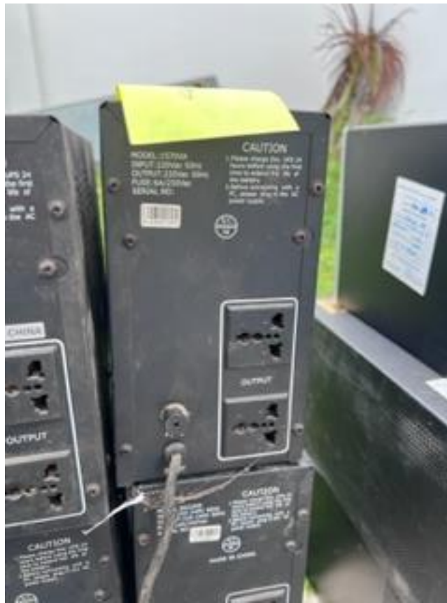
UNREADABLE UPS-BLUE GATE 1570VA
