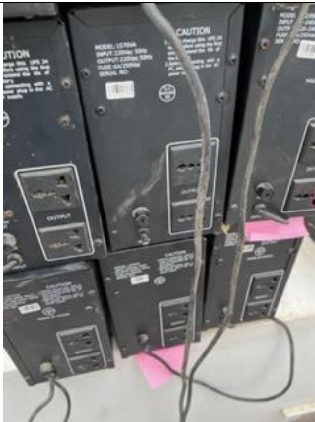
UNREADABLE UPS-BLUE GATE 1570VA
